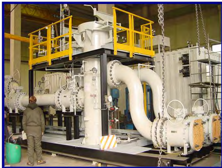
Package Gas Propane Filter
